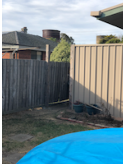
IMAGE OF WILFUL DAMAGE TO GATE: @ 1511 HOURS ON 9 MAY 2018
